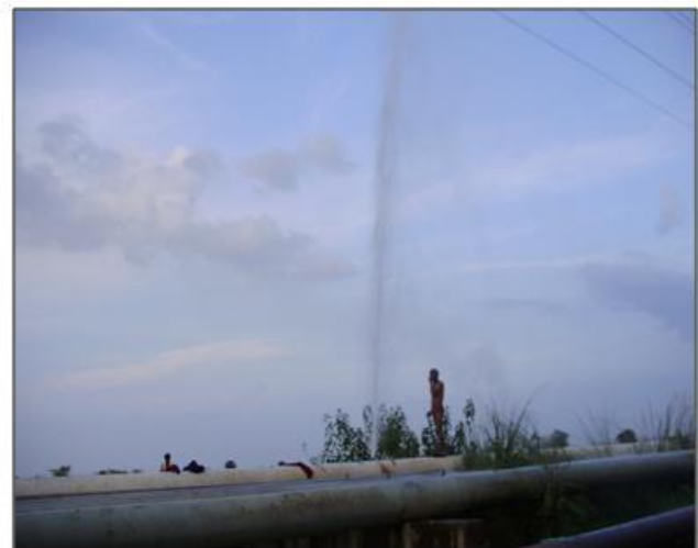
Leakage jet at pipe
