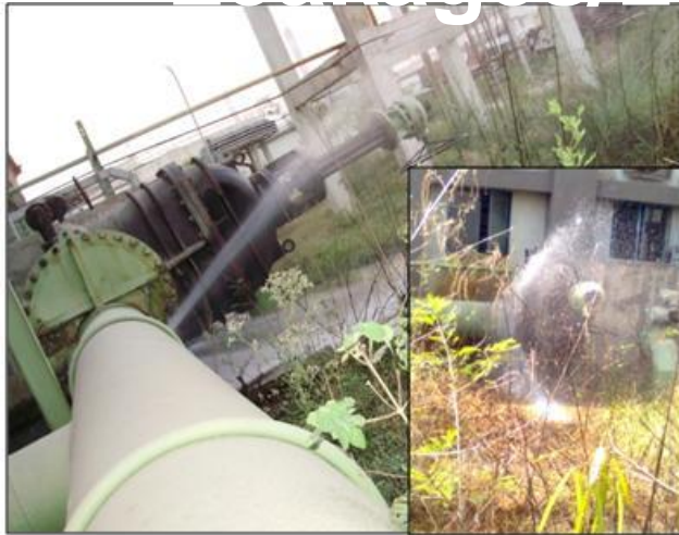
Leakage at pipe to aerator
