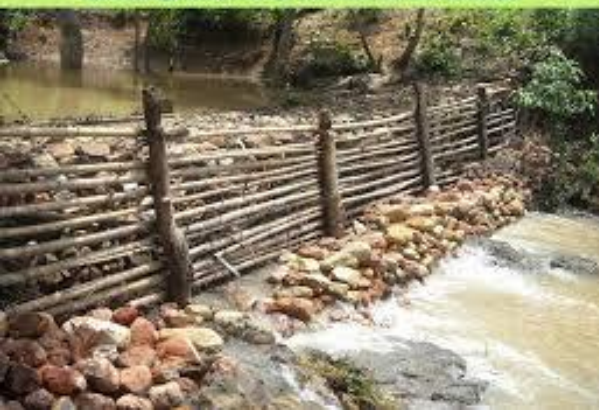
Series of loose boulder check dams with support of bamboo at East Singhbhum for prevention of soil erosion
