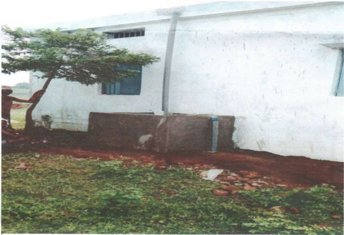
Roof Water Harvesting, Village-Pipariya,Block- Mohgaon, Distt.-Mandla.
