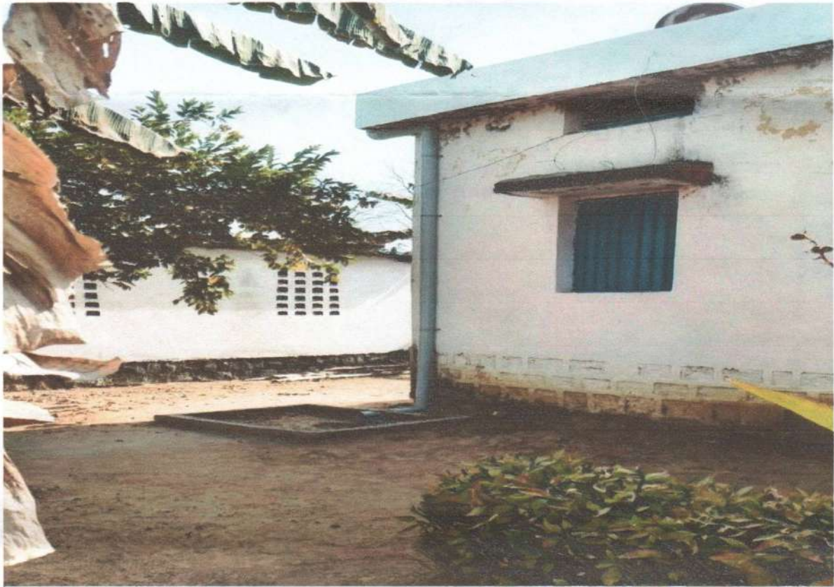
Roof Water Harvesting, Village-Kamta,Block- Nainpur, Distt.-Mandla.
