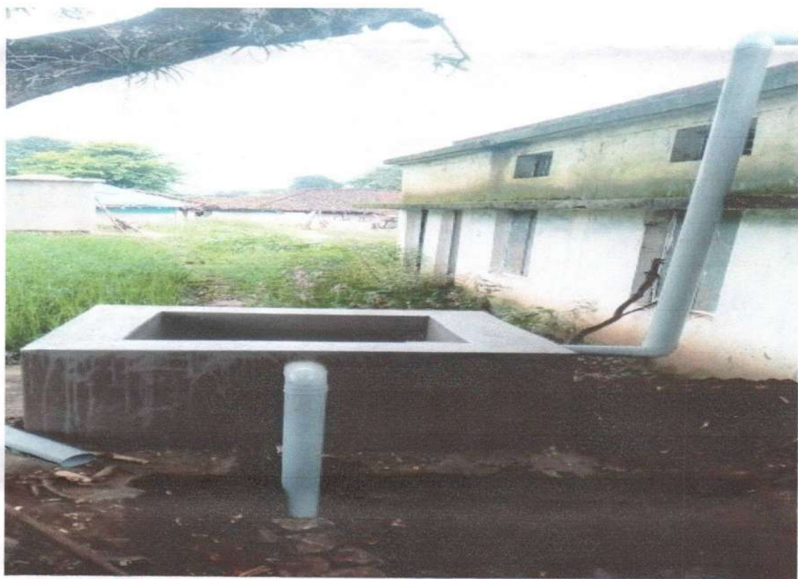
Roof Water Harvesting, Village-Singarpur, Block- Mohgaon, Distt.-Mandla.
