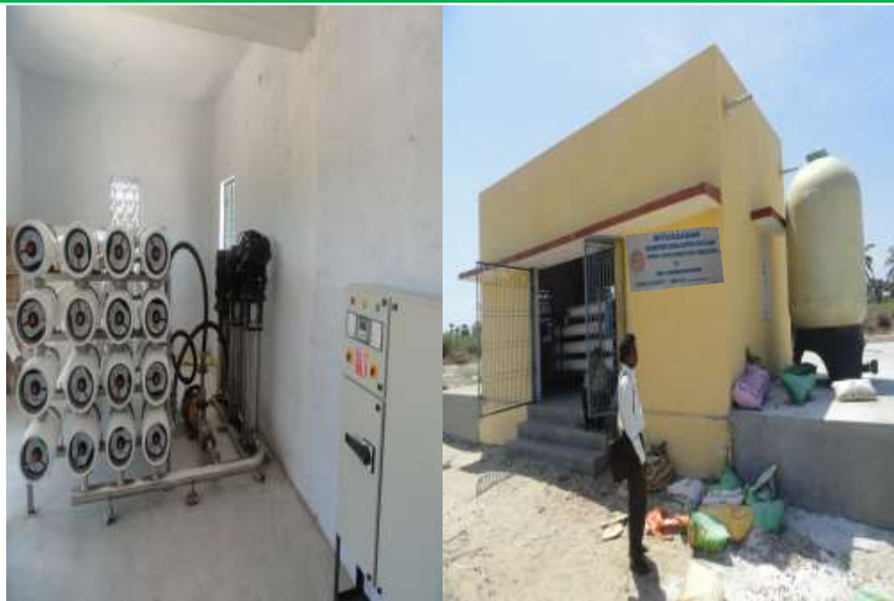
6000 LPH SEAWATER RO PLANT Village: Ervadi , Tamil nadu
