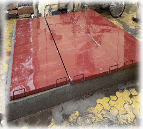
Recharge system Sarvodaynagar society
